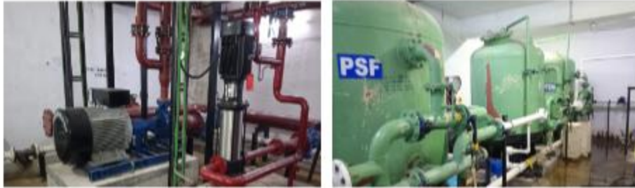
Figure 8. RO and water supply pump room
