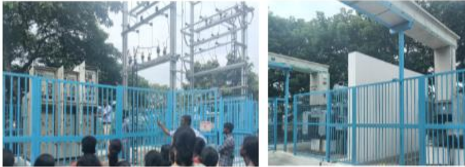
Figure 6. shows Step-up and stepdown transformer
