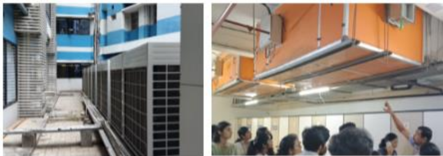
Figure 3. shows (a.) Outdoor compressor unit (b.) ceiling mounted Air Handling Unit
