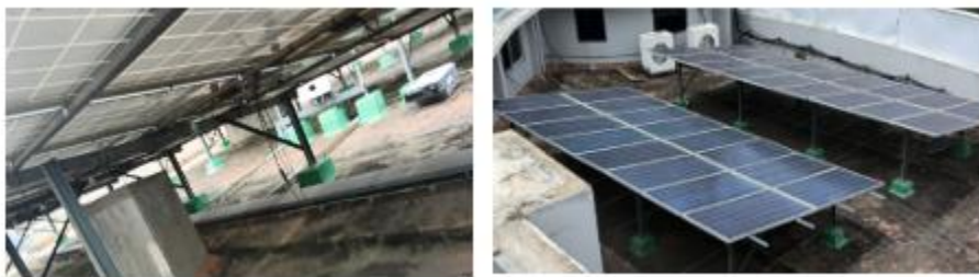
Figure 9. shows roof solar panels
