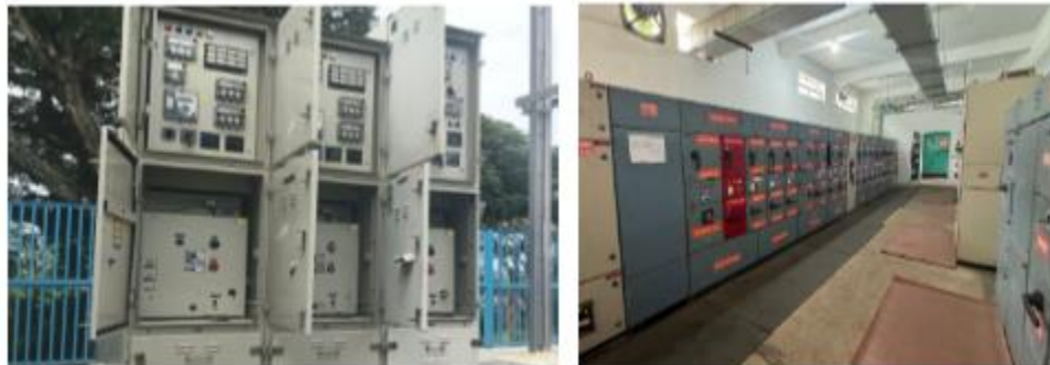
Figure 7. Circuit breaker and Circuit Board room
