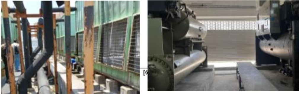
Figure 5. shows (a.) Cooling tower unit (b.) Condensor pump
