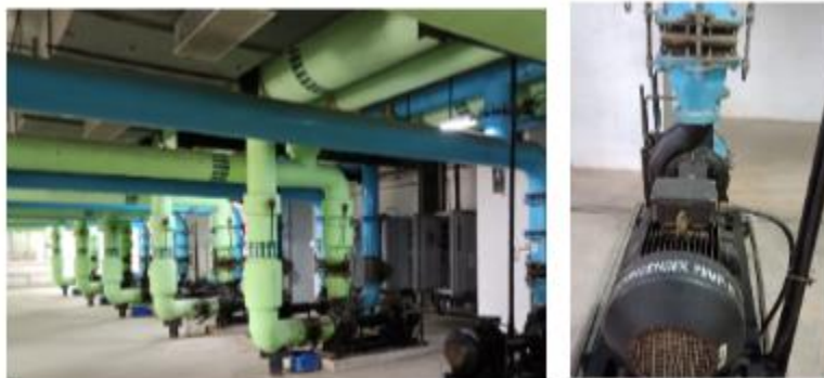
Figure 4. shows (a.) Chiller unit (b.) Condensor pump
