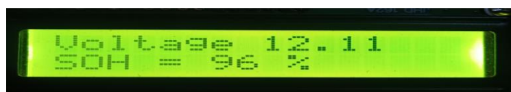
Figure (4) Voltage supply to the battery and state of health of the battery is displayed
