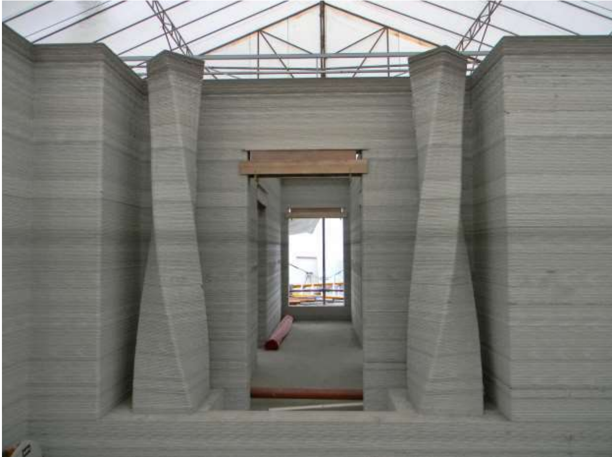
Fig.(10) Hotel Is 3D Printed from Sand and Volcanic Ash - Bing https://inhabitat.com/wp-content/blogs.dir/1/files/2015/09/Lewis-Yakich-3D-printed-hotel-suite-3-889x667.jpg their building which measures 10.5 m x 12.5 m (approximately 34.5 feet x 41 feet) in dimensions with a height of 3 meters (approx. 10 feet), making it about 130 square meters (1500 square feet). It is a two bedroom villa with a living room and jacuzzi room (with 3D printed jacuzzi), all of which will be part of the prestigious Lewis Grand Hotel. In all, the structure took approximately 100 hours of print time to complete, although the process was not a continuous one.
