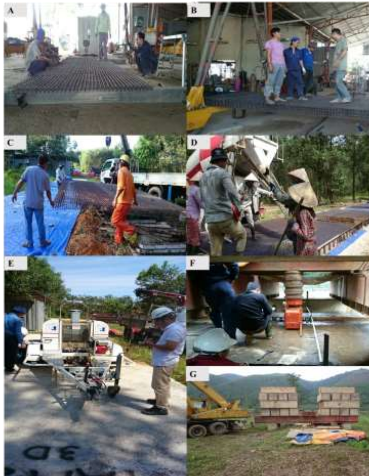
Fig. 1: Actual photos taken in the field: A, B, C. Installation of 3D wire mesh panels; D. 3D slab concrete pouring; E. Testing for load assessment by FWD device; F, G. Testing of destructive compression to determine calculation data.
