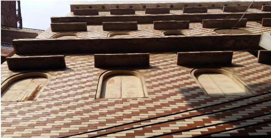
Figure 7 Low-rise apartment building in “Androon” Lahore, built in the 90’s, lacking any elements for ventilation except the windows that cannot be opened during the immense heat wave throughout most of the year. Taken by author, 2018.
