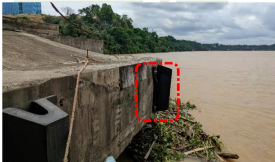
Figure 5. Condition of rubber fenders on pillar P4
