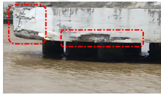
Figure 6. Concrete condition of pilecap at P3 pillar
