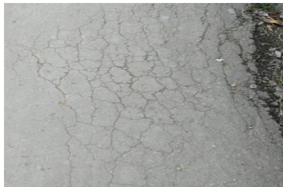
Fig. 12: Sample Alligator cracking
