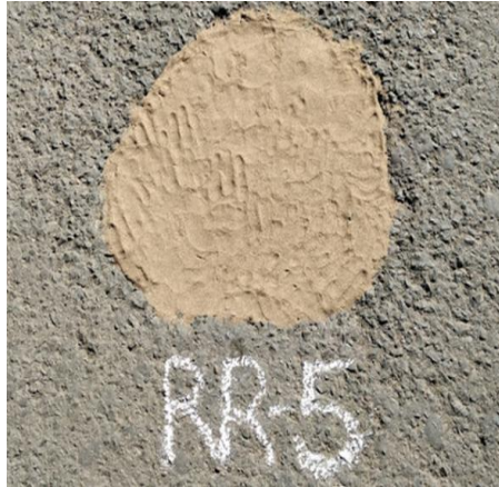
Fig. 8: Volume Determination by Replacing Sand with Bowl of Pothole
