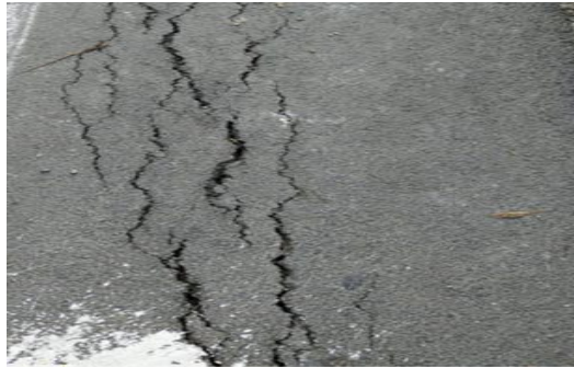
Fig. 10: Sample of Longitudinal cracking
